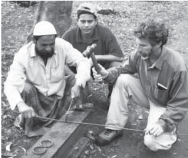
Alan with Dhaka Zoo staff fabricating "S" hooks for the hemp rope for the hoolock enclosure
